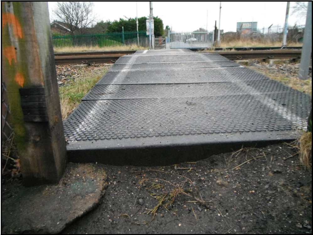
Figure 24: There is a significant trip hazard formed by the edge of the outermost deck panel. This edge is normally obscured by the closed gate which increases the likelihood of tripping. The overspill from the gate post concrete also presents a trip hazard to crossing users.
