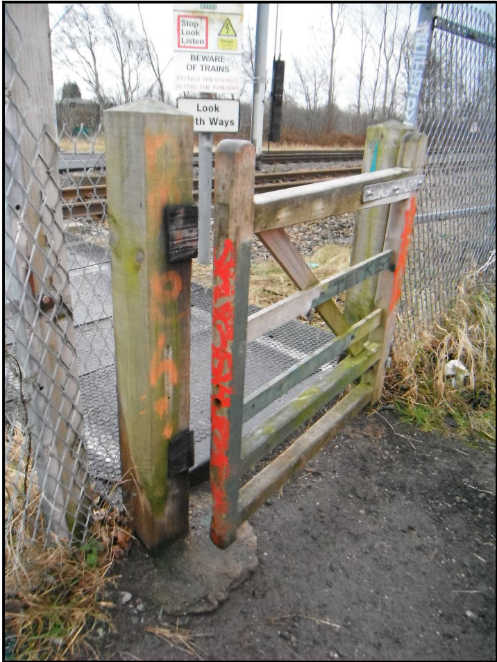
Figure 25: During strong winds it was noted that the access gate did not fully close, despite being self-closing. This has been reported to Network Rail (reference: 170213-000138). In light winds, the self-closing mechanism was found to work correctly.
