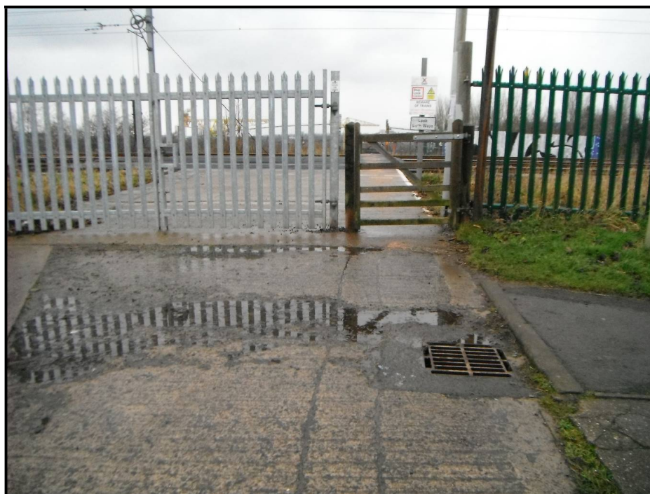
Figure 13: Despite the provision of a drainage gully, surface water pools on the entrance to the crossing. In freezing temperatures, this will become icy and result in hazardous underfoot conditions. There is a Road/Rail Access Point (RRAP) adjacent to the crossing gate. It is assumed that the RRAP will only be utilised with the appropriate safe system of work, therefore the increased risk to crossing users is thought to be negligible. As confirmed with David Guy (Network Rail Level Crossing Manager) on 17 th February 2017, the RRAP is for the use of Nexus staff only as no vehicular deck is present on the Network Rail freight line.
