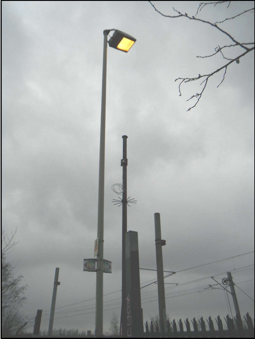
Figure 11: South Drive Footpath Level Crossing is illuminated by lighting provided by the railway. It appears to be sodium based lighting. The lux levels across the deck were not tested during the site visit so it is unknown whether the existing level of illumination is compliant across the whole footway surface.
