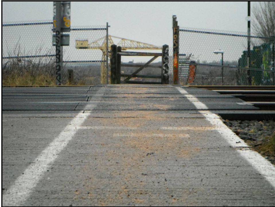
Figure 18: Temperatures on the day of the site visit were very low. The crossing surface had been recently salted which gives a good indication of regular maintenance attendance. It may also point to a history of hazardous underfoot conditions in freezing temperatures. The white lining over the deck itself on the left side of the photo is beginning to wear off. It is not clear who is responsible for salting the deck, an operation which in itself is presumably subject to an agreed method of working.
