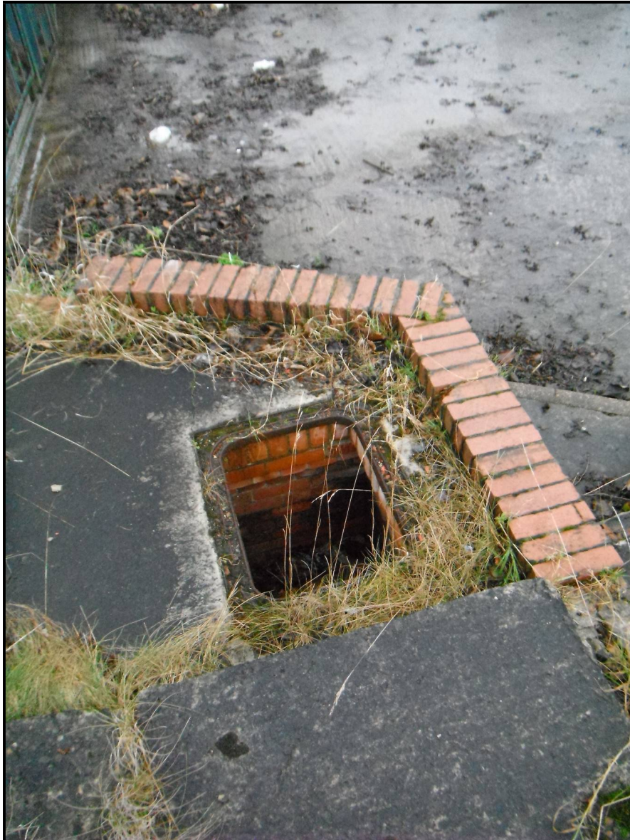
Figure 9: A manhole cover was missing in the south east corner of the crossing – although members of the public are unlikely to utilise this area, there is still a significant risk of physical harm to members of the public. This was subsequently reported to South Tyneside Council via their website reporting system.
