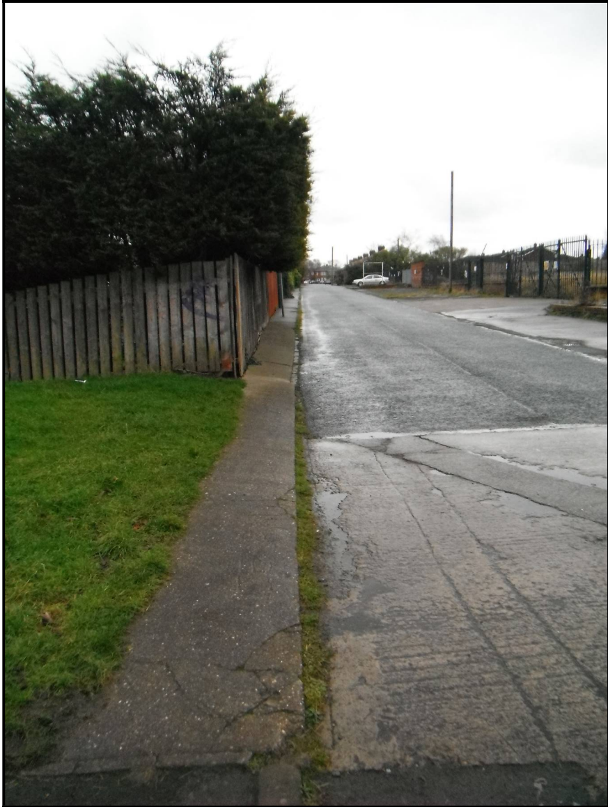
Figure 12: The designated footway on South Drive is of concrete construction and slopes towards the carriageway. It is also overhung by trees from the adjacent property, reducing available head room to pedestrians. Both of these factors contribute to forcing pedestrians to walk in the carriageway.
