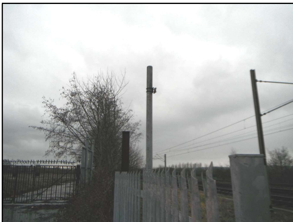
Figure 14: There is evidence of a previously installed height gauge above the RRAP – presumably to provide a safe height for vehicles due to the presence of existing overhead electrification equipment. There is an existing post and bracket installed on each side of the vehicular access
