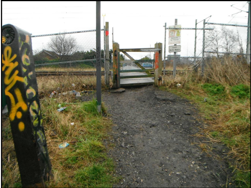
Figure 26: The immediate approach to the crossing is un-metalled, uneven and slopes down towards the river. There is an increased likelihood of slips, trips and falls for members of the public.
