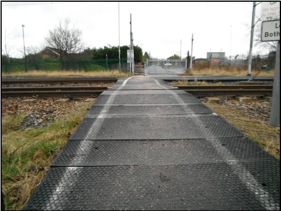
Figure 22: Holdfast deck panels are installed up to the crossing gate on the Riverside Park side of the crossing. The surface is anti-slip but it is uneven and the edges of the panels present a trip hazard to users. The footway appears to be of sufficient width (based on the width of the crossing gates) with sufficient distance from the white lining to the edge of the deck surface. However, the white lining that demarcates the footway and the decision point is beginning to wear off.
